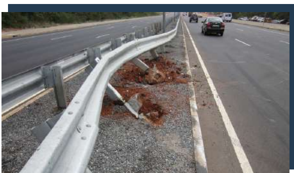
Damaged or Missing Barricades
